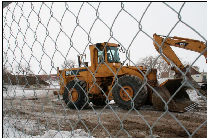
Tractors remove contaminated dirt from the plume site where the old refinery once was. Several empty lots and the intersection will have dirt treated as part of the cleanup process.
